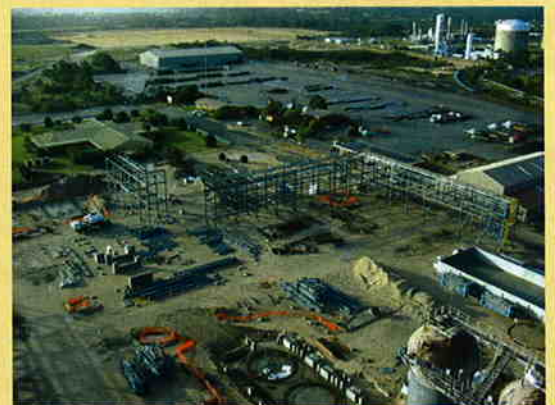
Under way: After 20 years of planning, Rio Tinto's revolutionary A$400 million Hismelt pig iron plant is now rapidly taking shape on the Kwinana industrial strip south of Perth.
